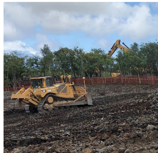
Construction crews work at the site of the Kaloko Heights Affordable Housing Project.
