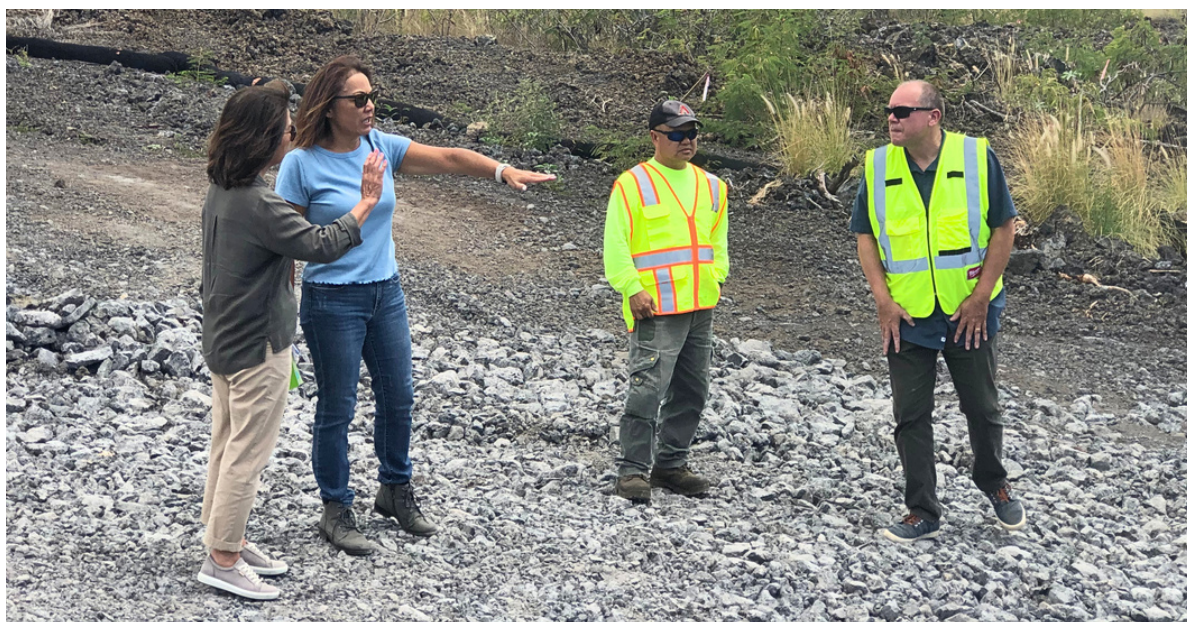
County of Hawai'i Office of Housing and Community Development Housing Administrator Susan Kunz (far left) and Community Engagement Division Manager Sharon Hirota (left) get an update on the Kukuioala Emergency Shelter and Assessment Center from contractors during a recent site visit.
