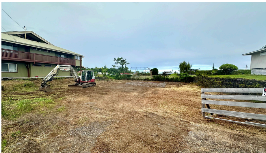
HALE O Hawai'i County Community Land Trust started work this month on single-family homes in Hilo and Volcano fully funded by the County's Affordable Housing Production Program (FY 2023-24). Pictured above is the future site of one of these homes on State-owned land conveyed to the County by an executive order then leased to HALE O Hawai'i as part of a pilot project that will provide a template for development of single-family affordable housing on State-owned lands under a land trust model. Once complete, the homes will be sold to eligible purchasers under a long-term generational leasehold in which immediate family may inherit the lease. For more information on HALE O Hawai'i, please visit https://haleohawaii.org . Courtesy photo
